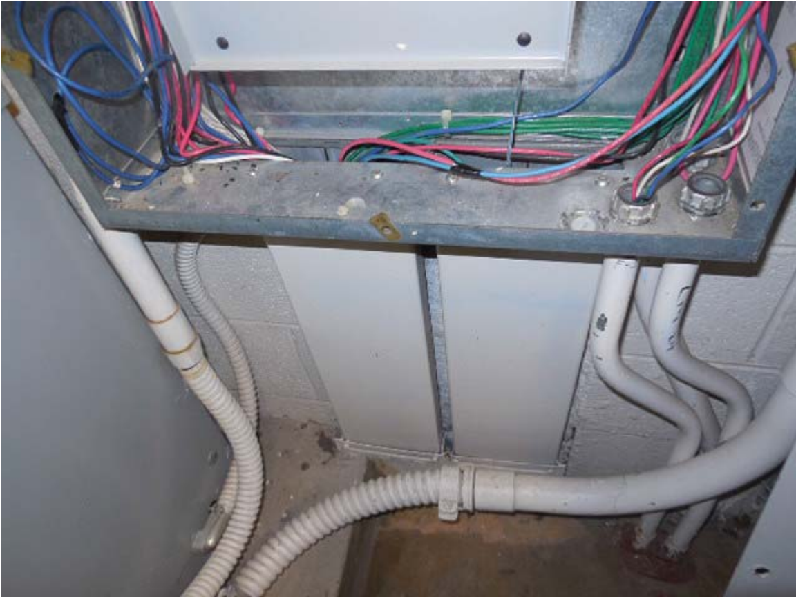
Picture 11: C10 Reagan Airport North – Panel F – Ducts below Panel
