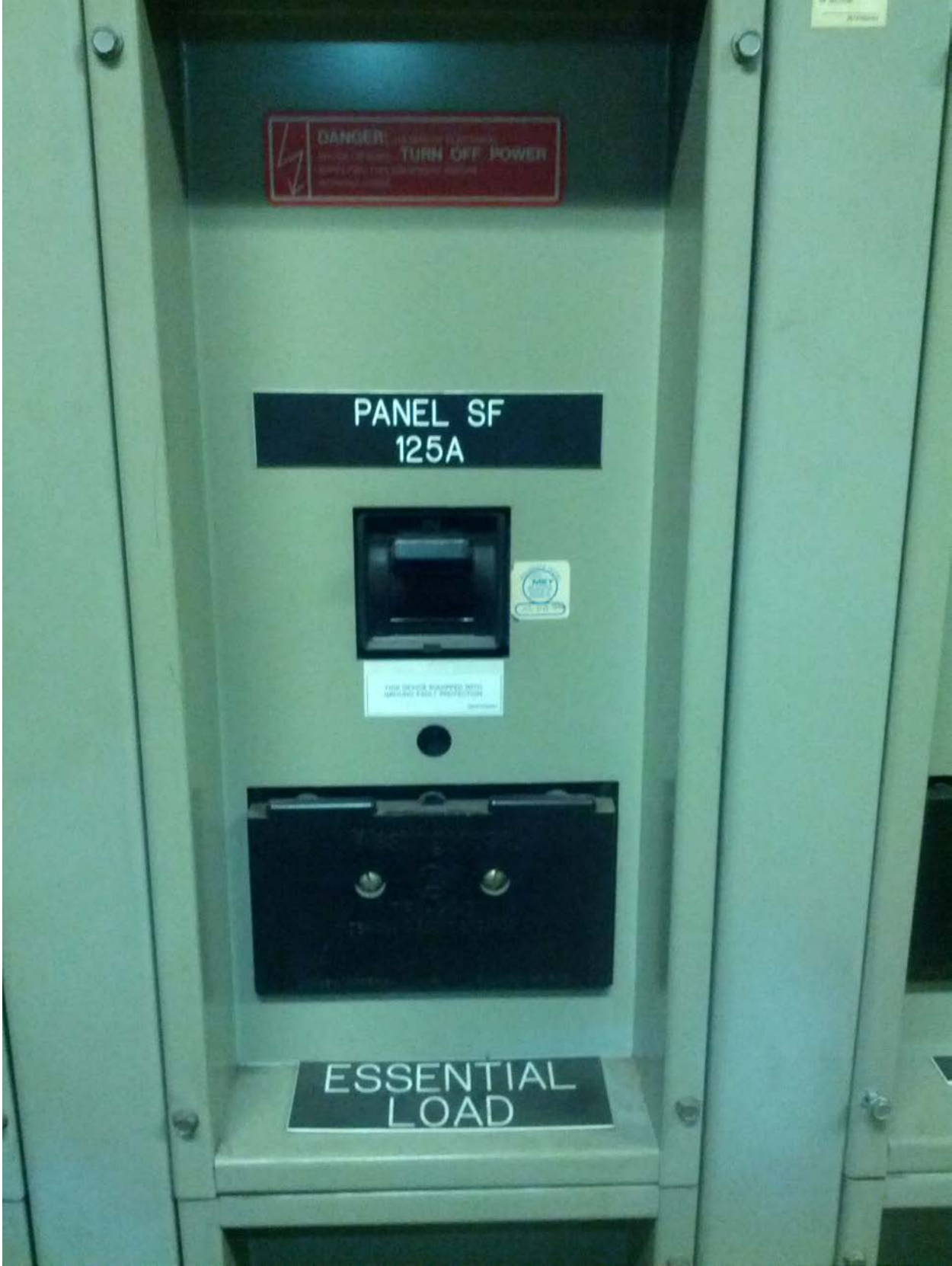
Photo #11: E02 Shaw-Howard U (South) – SWBD Breaker for panel SF
