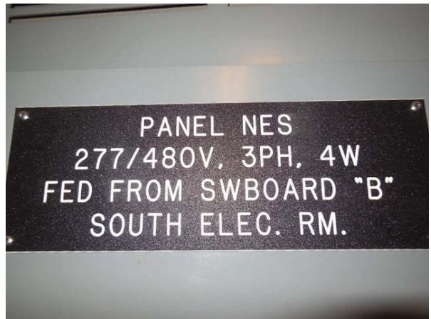
King Street North Photo #6 – Panel NES which feeds Panel NESS Panel Schedule- Electrical Room #N201
