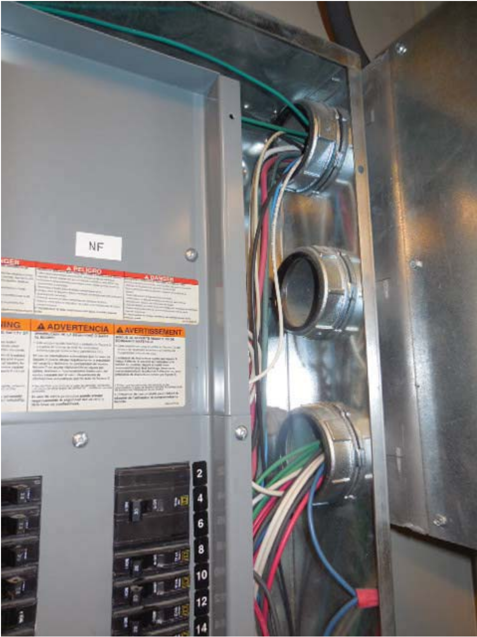
King Street North Photo #3 – “Panel NF” Side Feed Conduits into Shared Trough - Electrical Room #N201
