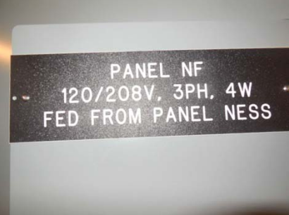
King Street North Photo #1 – AFC Panel NF located in Electrical Room #N201
