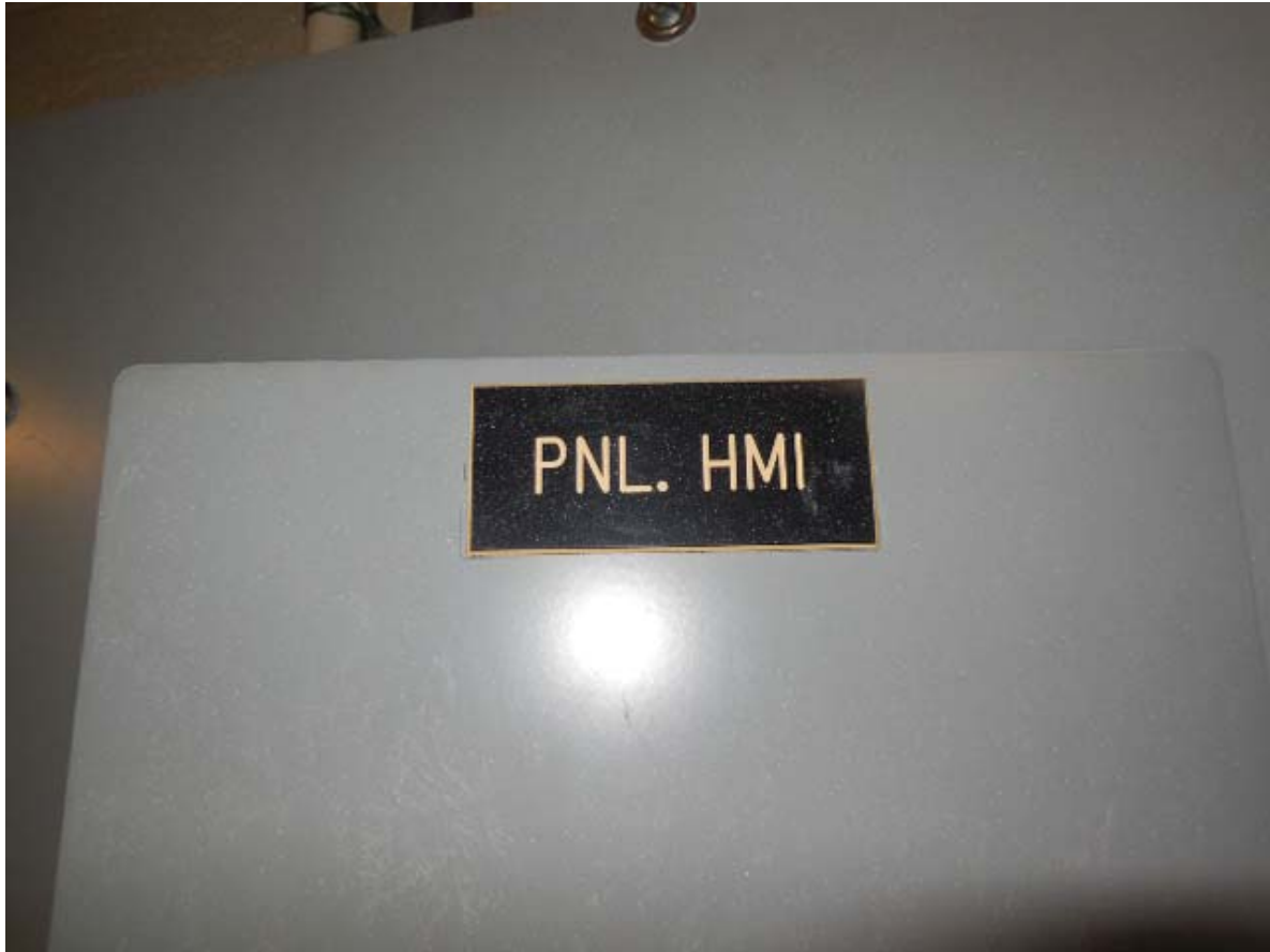
Picture 12: C10 Reagan Airport North – Panel HM1 in Room 119
