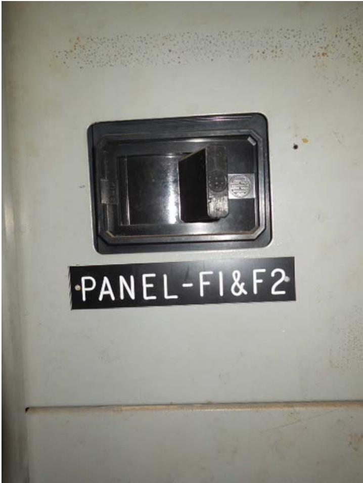
Photo #8: C13 King Street (South) – Switchboard circuit label for Panels F1 and F2
