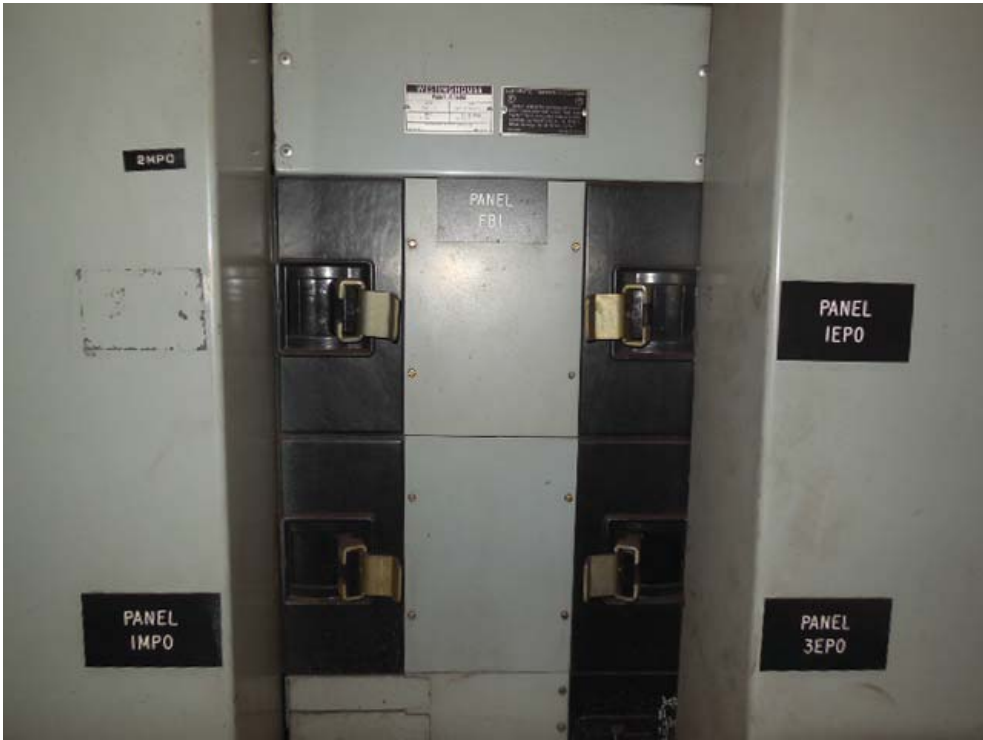
Photo #10: C09 Crystal City – Source breakers on Panel FB1 for panels feeding into common trough
