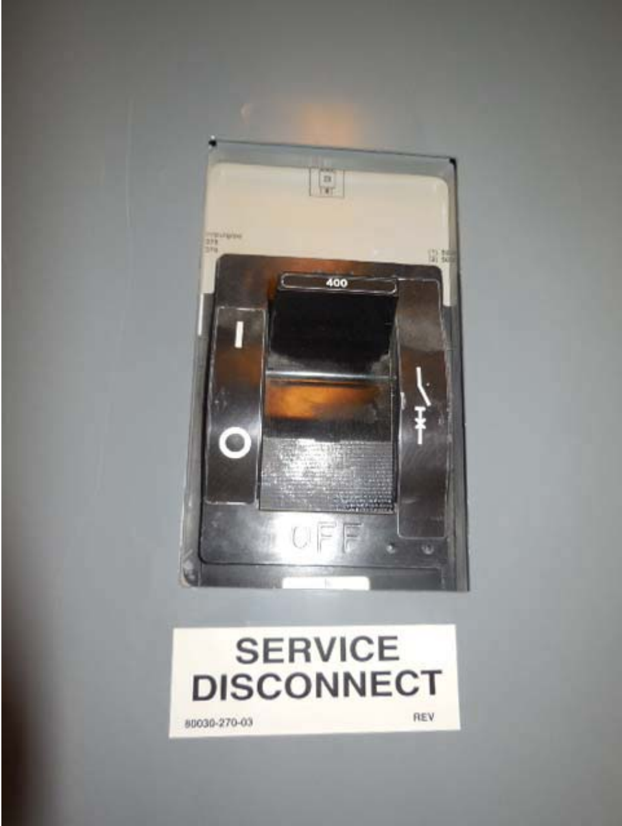
King Street North Photo #7 – Panel NES Main Breaker (Service Disconnect) used to de-energize Panel NES, Panel NESS and AFC Panel NF as all three panels share trough.
