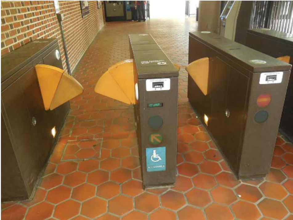
Photo #6: C13 King Street (South) – Mini-mezzanine mezzanine faregate array and floor handhole
