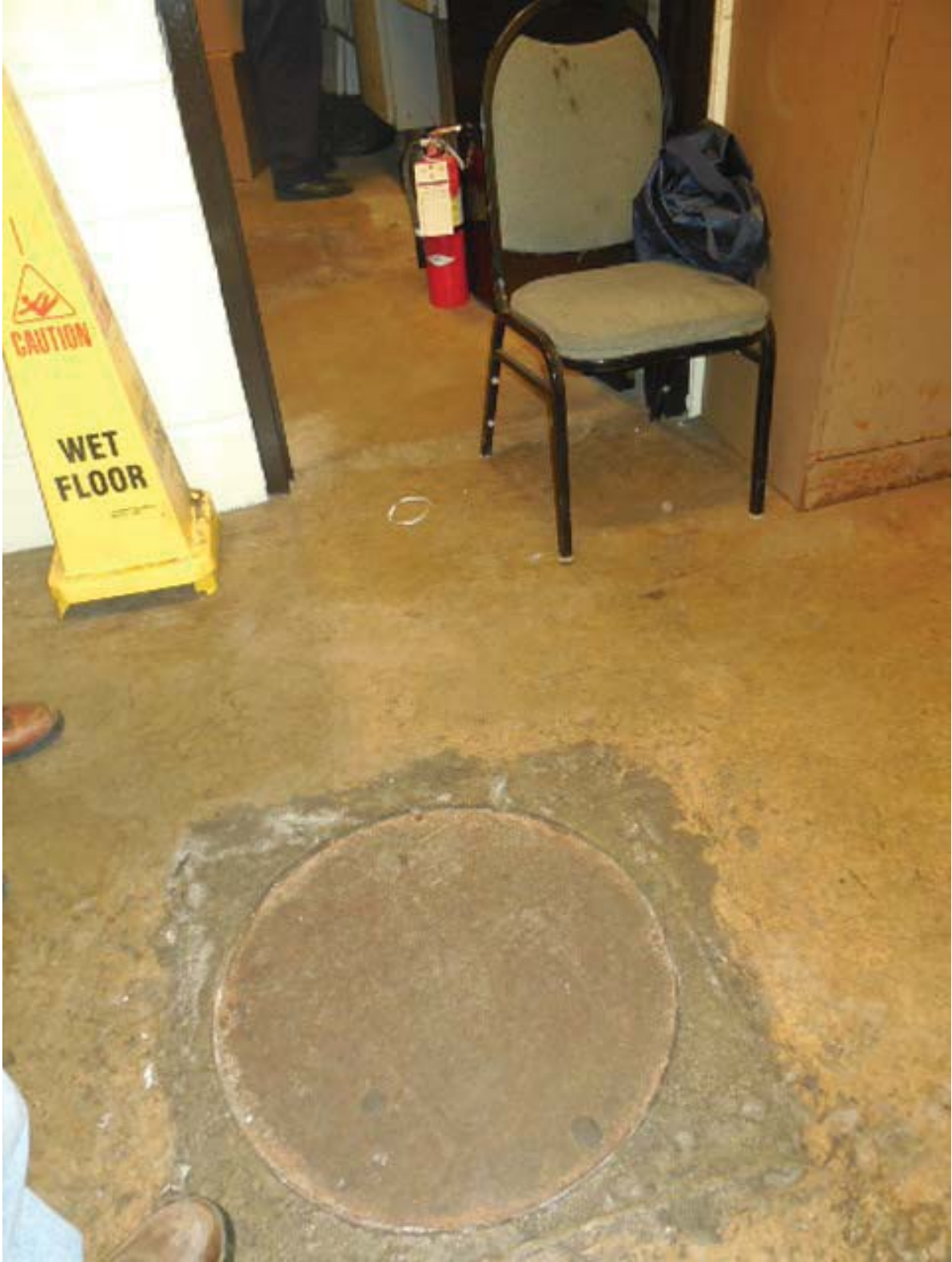
Mt. Vernon Photo #6 – Manhole located in hallway of C204 in which walker duct runs through to another manhole in mezzanine area by kiosk. About 81’ from AFC Panel (F).
