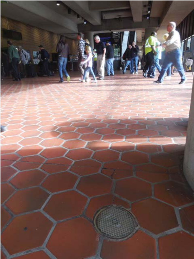
Photo #2: C12 Braddock Road – Handhole in Mezzanine area
