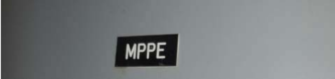
Mt. Vernon Photo #4-- AFC Source Panel (MPPE) located in Room #C207 on Mezzanine Level. Source Breaker (Circuit #4, 3PH) for AFC Panel (F)
