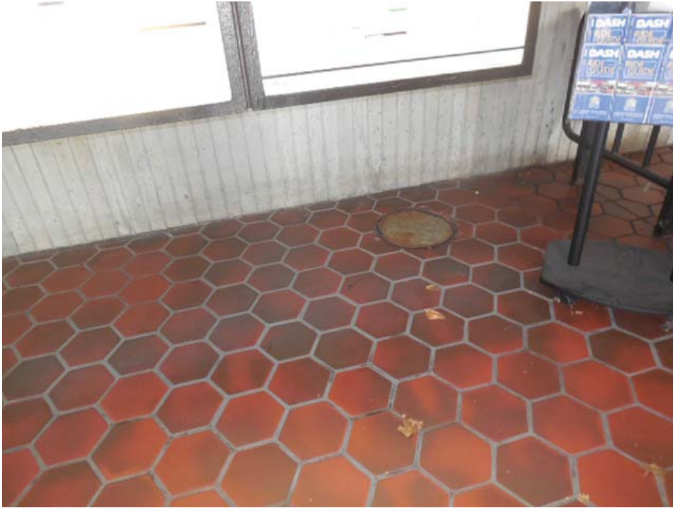
Photo #3: C13 King Street (South) – Handholes in mezzanine floor
