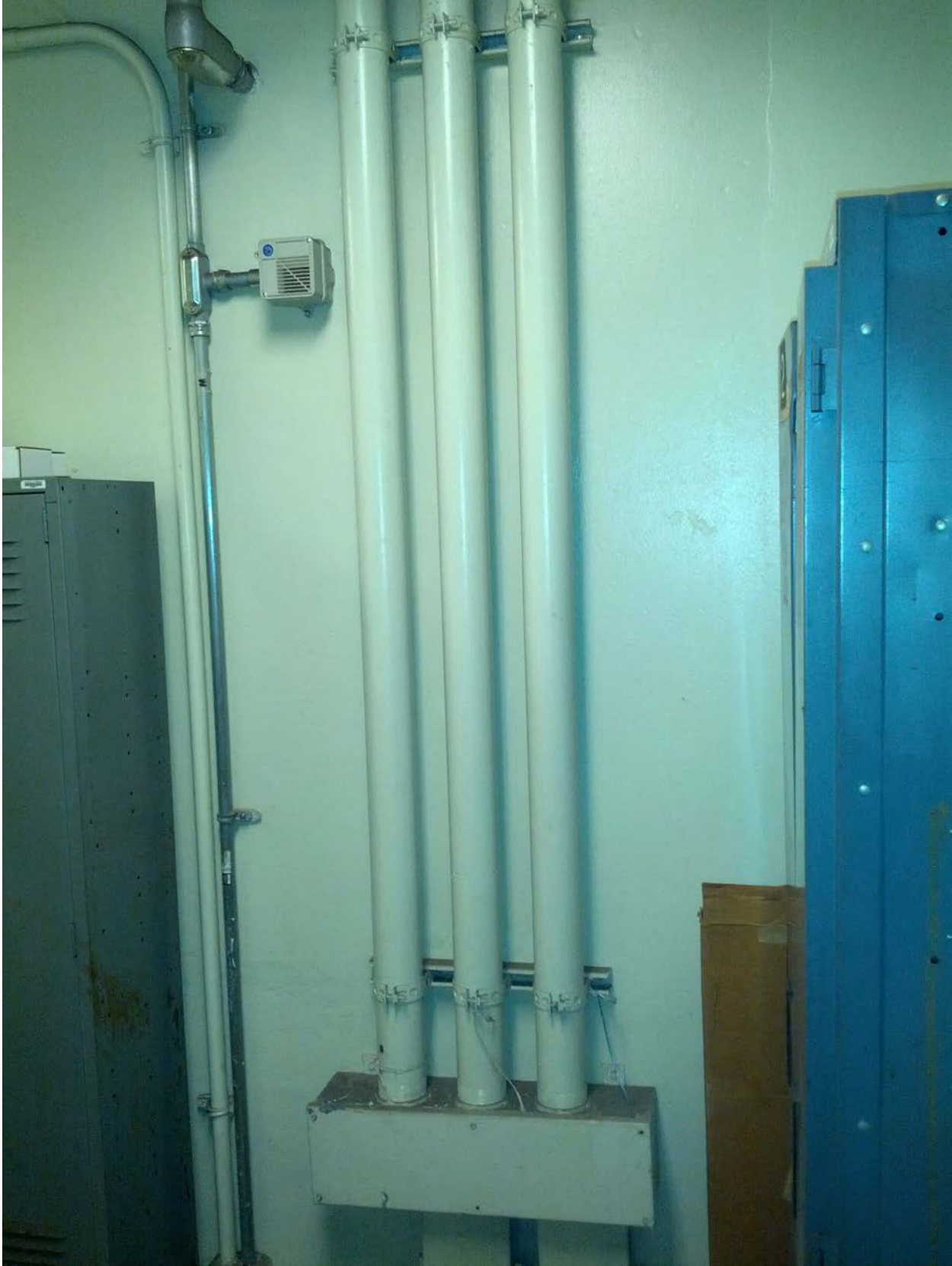
Photo #6: E02 Shaw-Howard U (South) – Conduit Riser near Room 208
