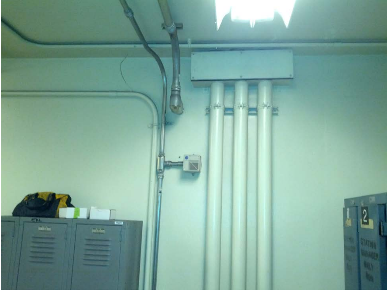
Photo #4: E02 Shaw-Howard U (South) – Junction Box and Riser near Room 208
