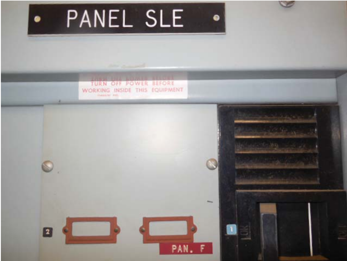
Photo #3: C10 Reagan Airport South – Panel SLE in Room C116
