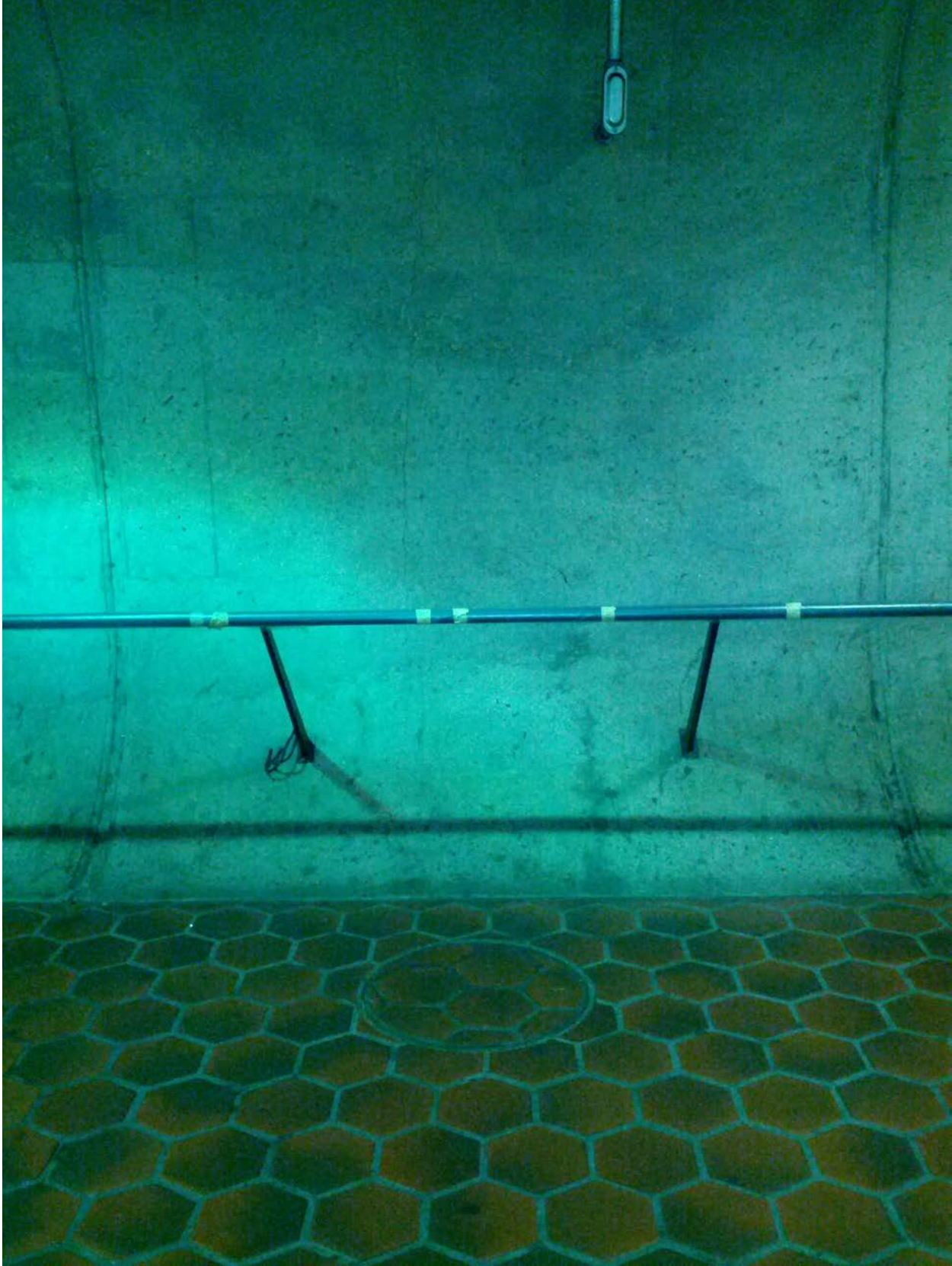
Photo #7: E02 Shaw-Howard U (South) – Mezzanine level handhole opposite Room 208
