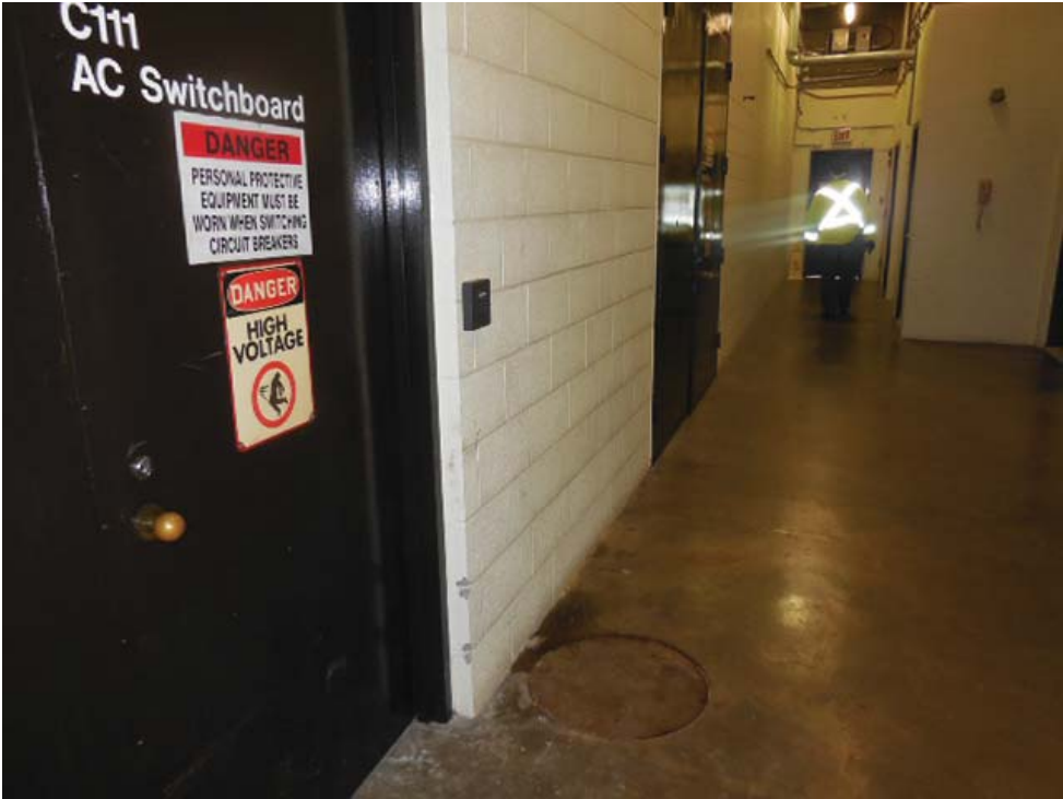
Photo #3: C12 Braddock Road – Handhole in corridor
