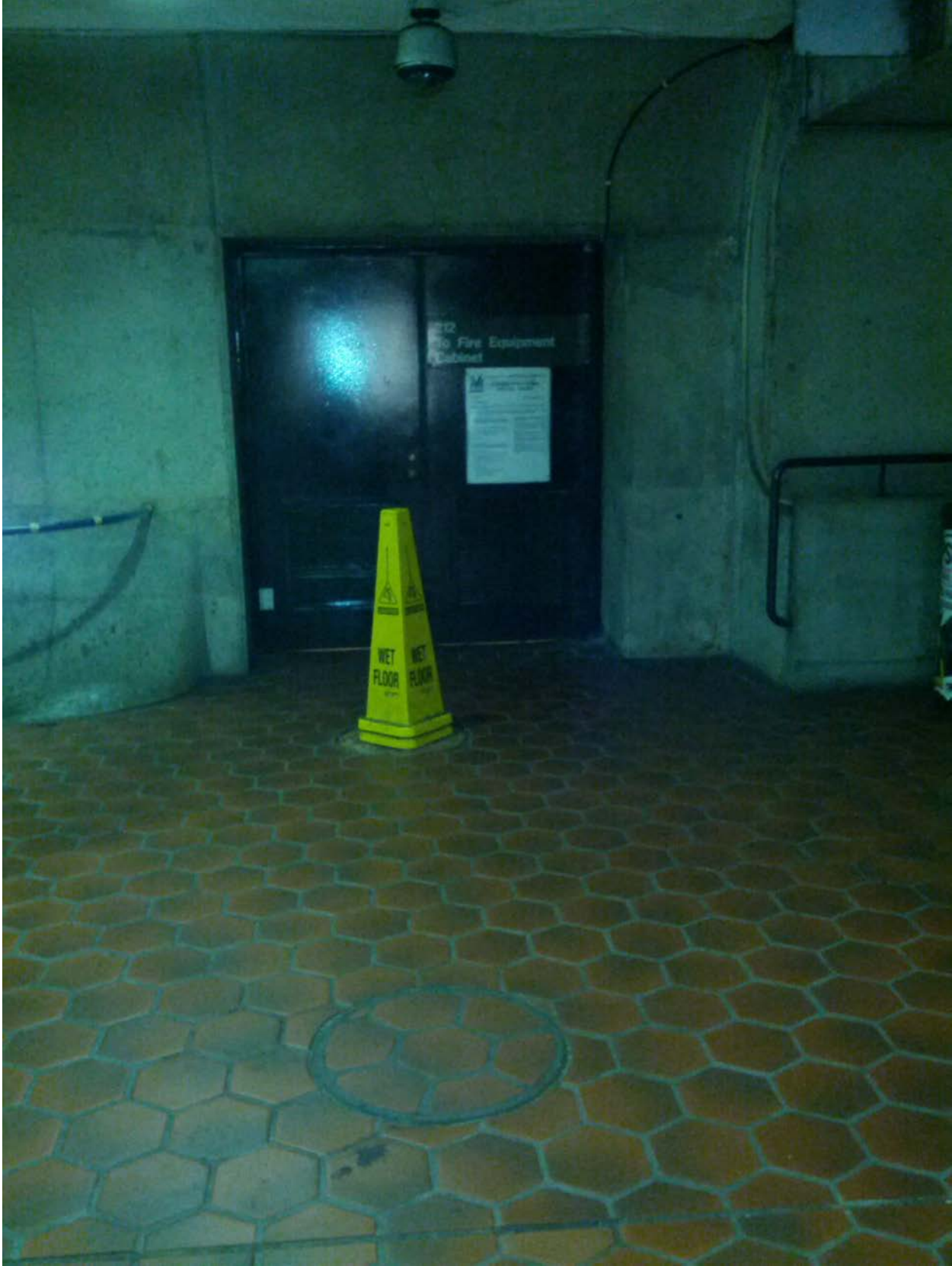
Photo #8: E02 Shaw-Howard U (South) – Mezzanine level handhole
