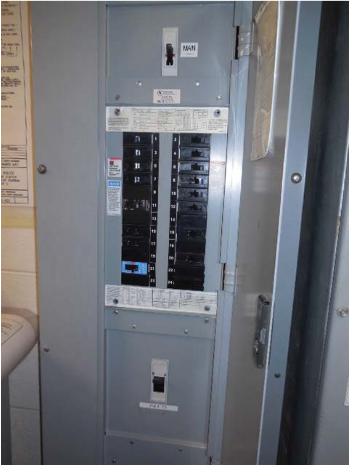
Picture 13: C10 Reagan Airport North – Panel HM1 in Room 119
