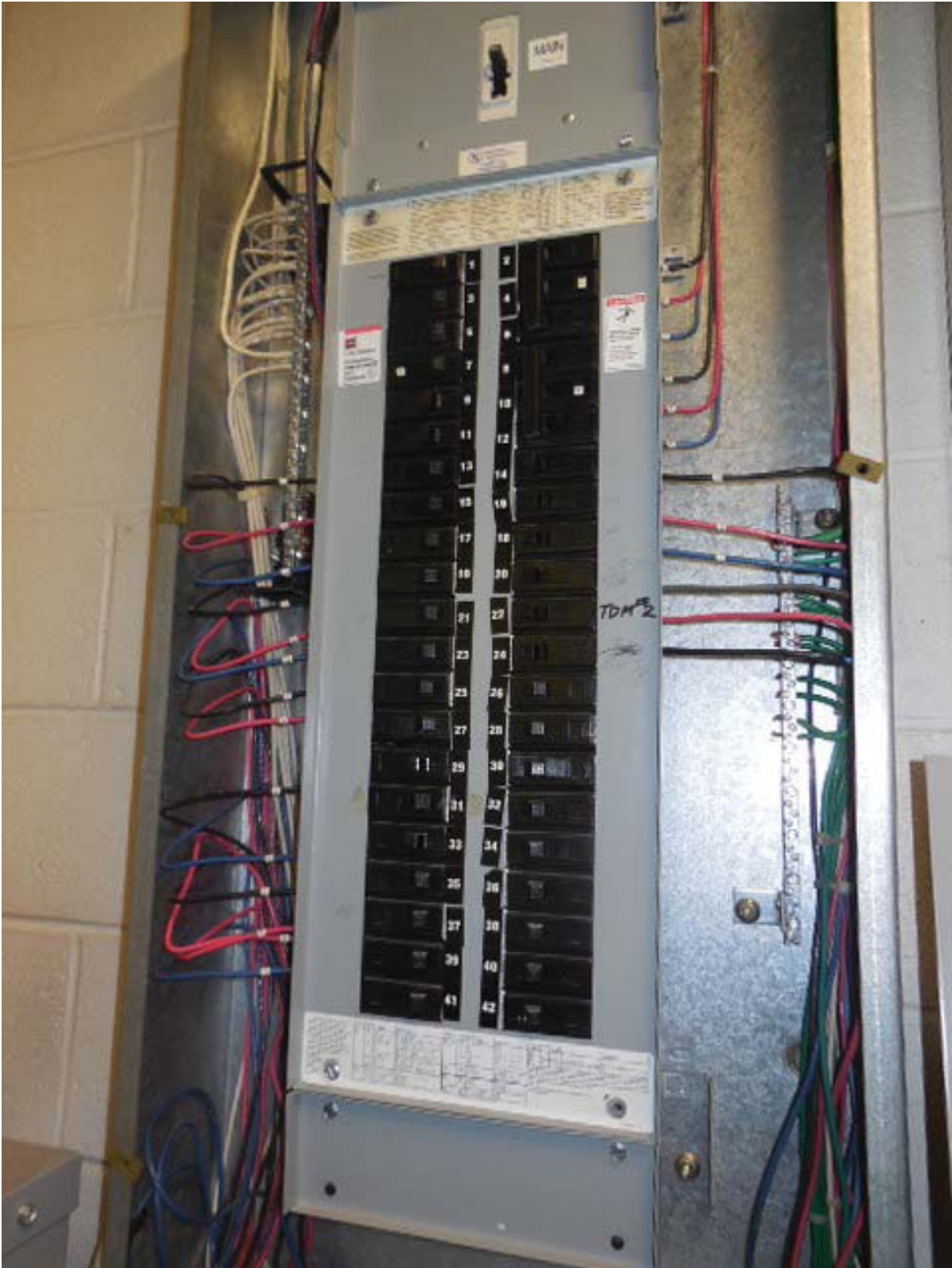
Picture 9: C10 Reagan Airport North – Panel F in Room 119
