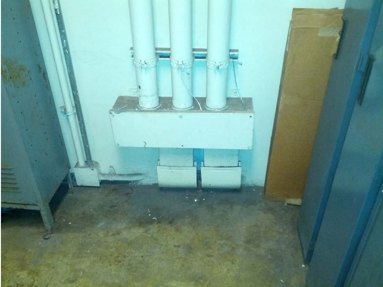
Photo #5: E02 Shaw-Howard U (South) – Junction Box, riser, and walker duct near Room 208
