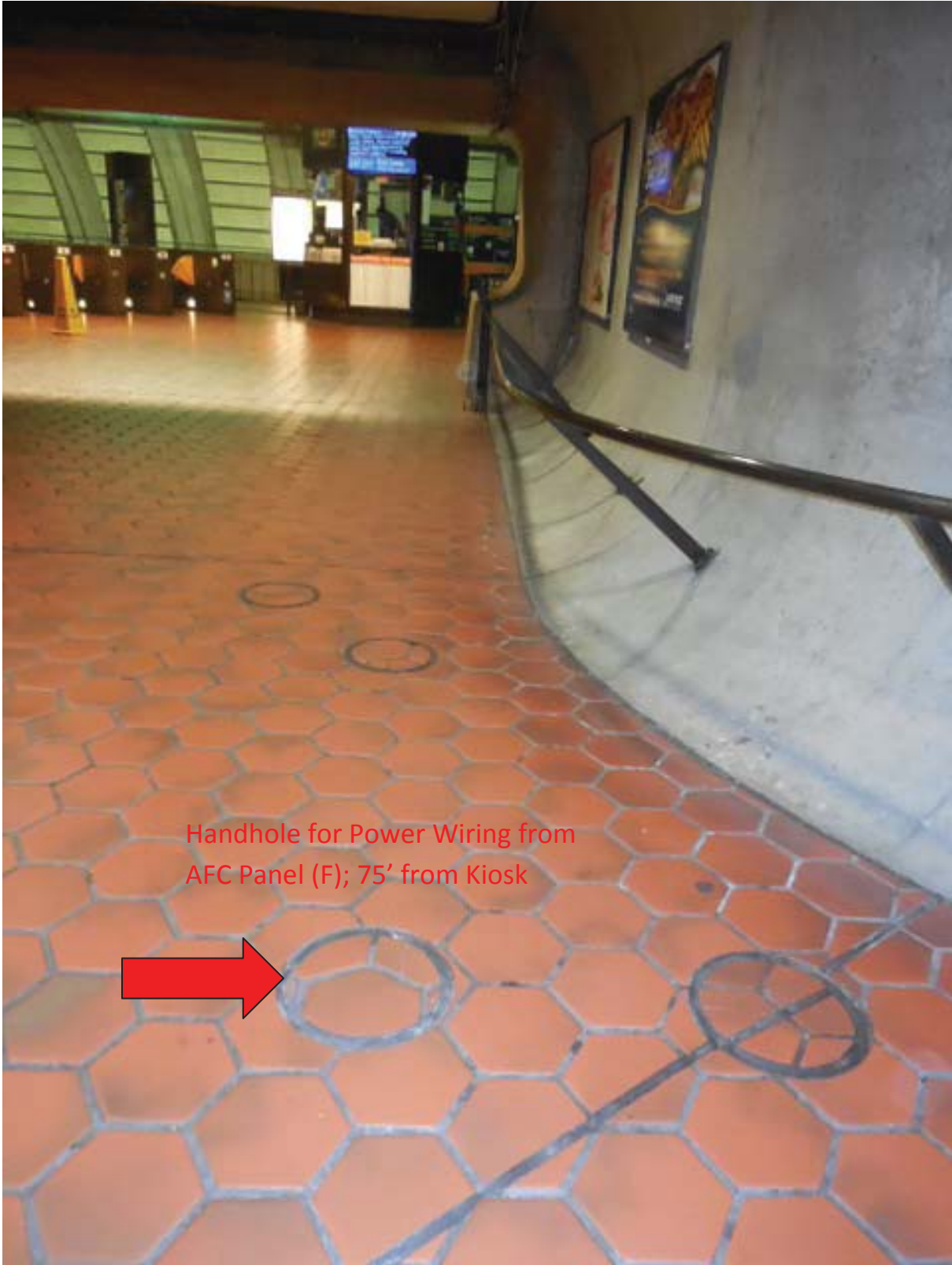
Mt. Vernon Photo #7 – Handholes located in mezzanine area by kiosk. About 75' from Kiosk.
