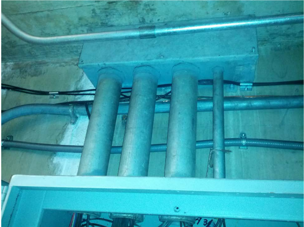
Photo #3: E02 Shaw-Howard U (South) – Junction box and drop to Panel SF in Room 208
