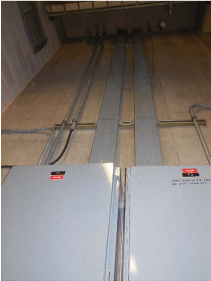
Photo #9: C13 King Street (South) – Ducts and conduits into panels F1 and F2 in Room C103
