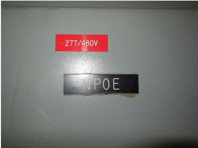
Photo #4 & 5: C15 Huntington North – Panel NPOE in Room 129
