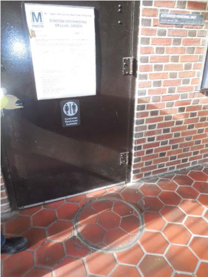
Photo #7: C13 King Street (South) – Handhole in mezzanine floor
