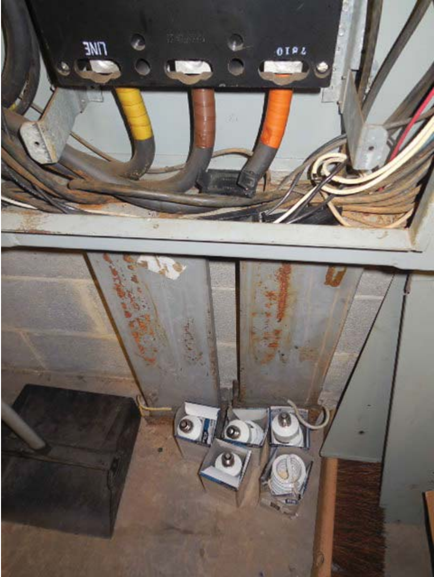
Photo #4: C12 Braddock Road – Ducts to Bottom of Panel F in Room C111
