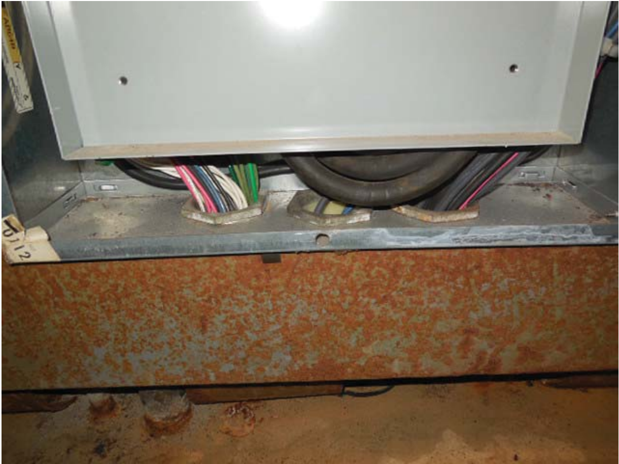
Photo #8: C15 Huntington North – AFC Panel NF – Ducts below Panel
