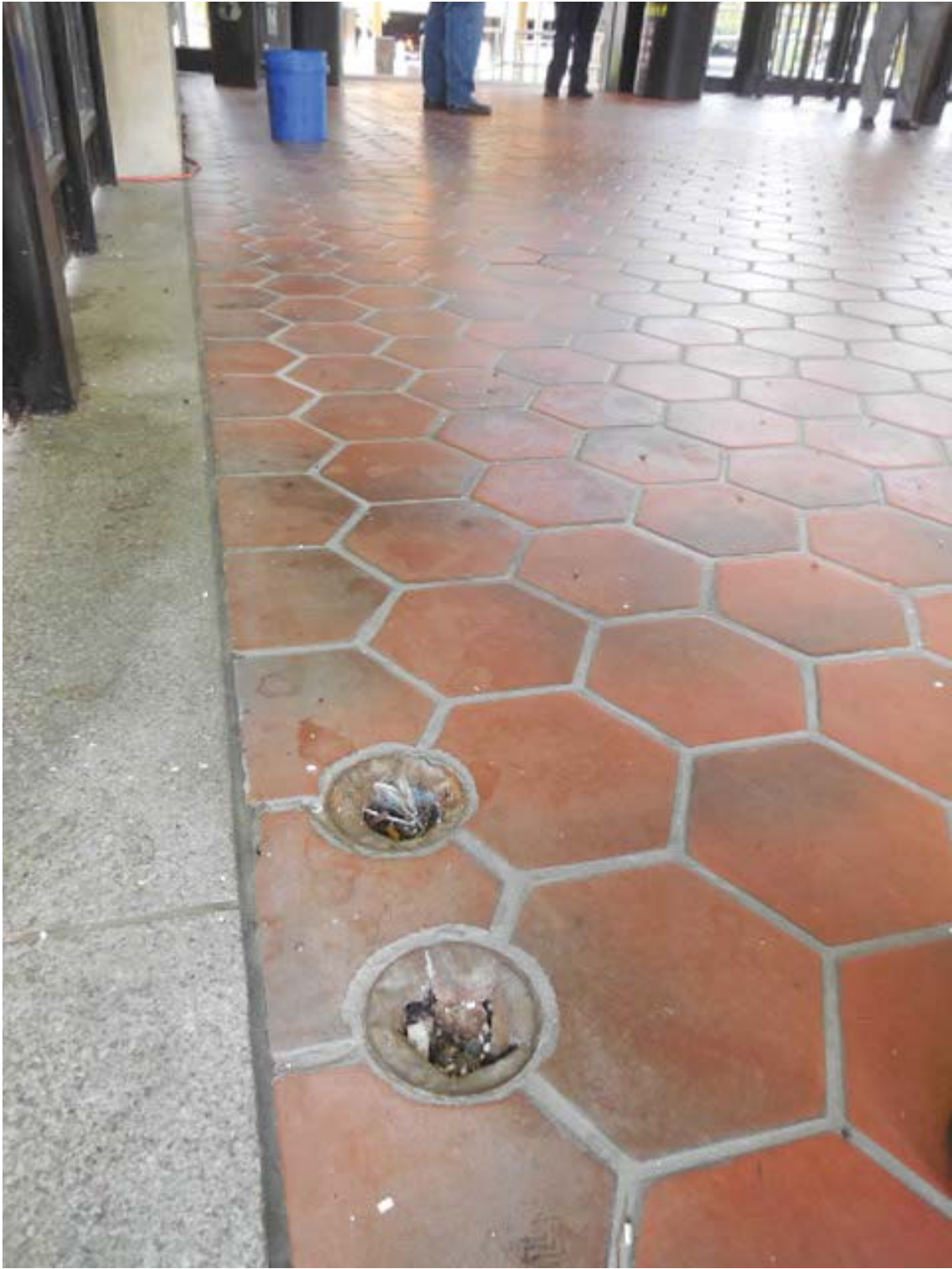
Picture 4: C10 Reagan Airport North – Handholes at Mini-Mezzanine
