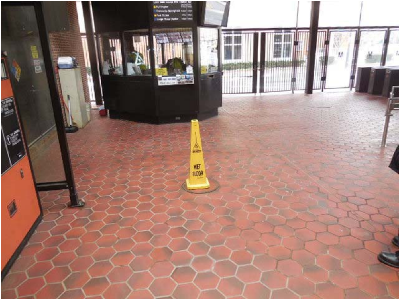
King Street North #9 – Handhole in Mezzanine Area used for Routing of Power Conductors from AFC Panel to Kiosk
