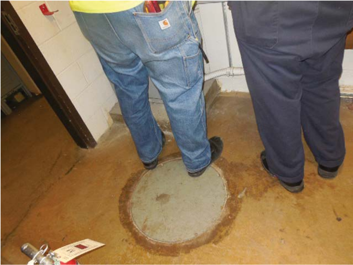
Picture 7: C10 Reagan Airport North – Handhole in Room 119
