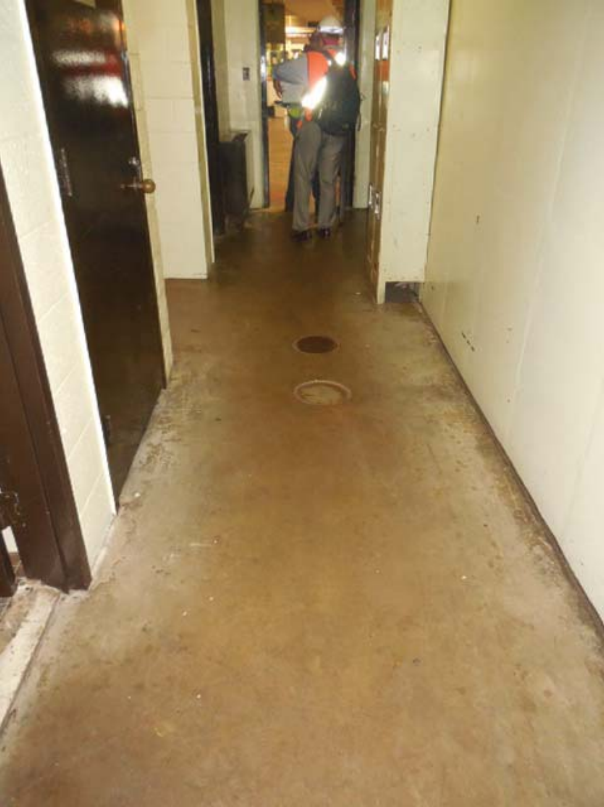
Photo #2: C10 Reagan Airport South – Handholes in hallway to Station Facility Rooms
