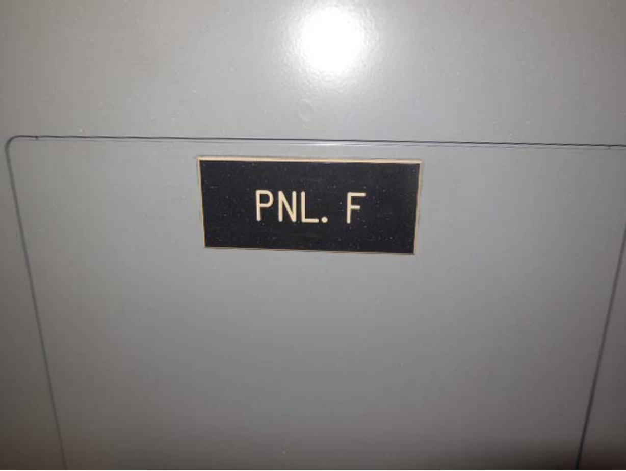
Picture 8: C10 Reagan Airport North – Panel F in Room 119
