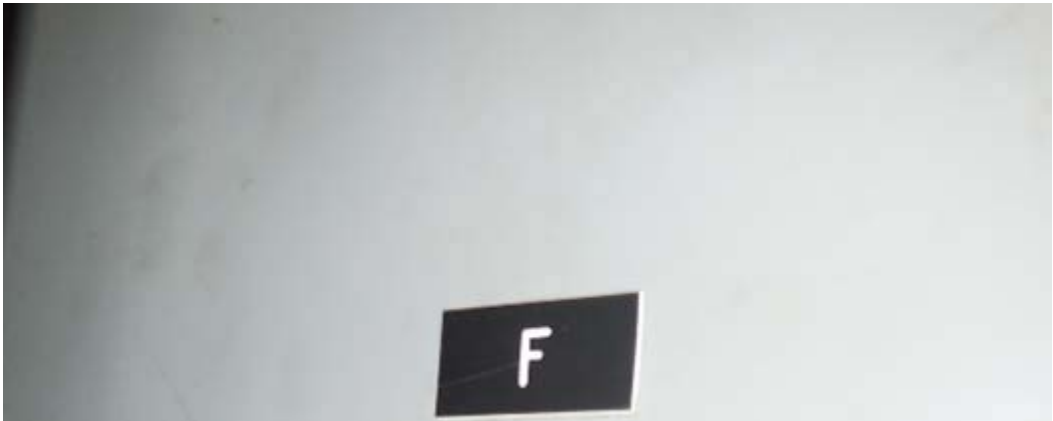
Mt. Vernon Photo #1 – AFC Panel (F) - Room C207 (Mezzanine Level)
