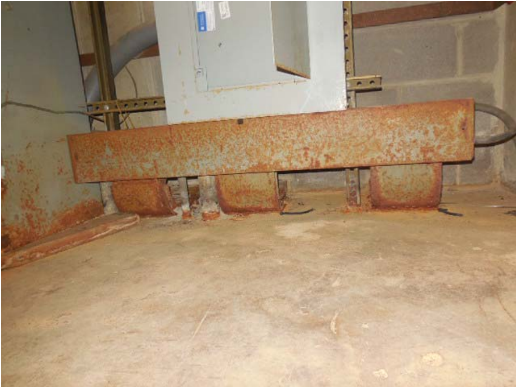
Photo #9 & 10: C15 Huntington North – AFC Panel NF – Bottom of Panel
