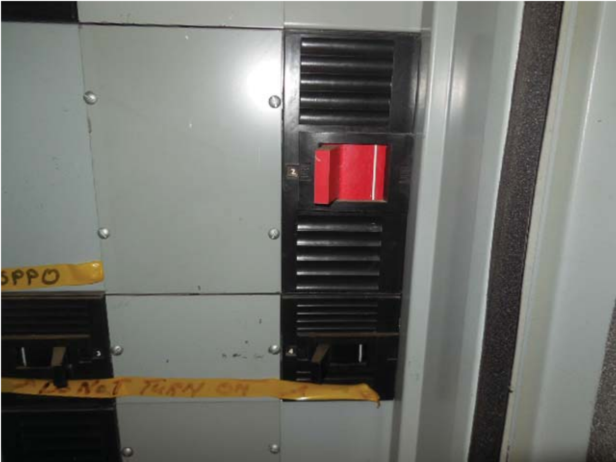
Photo 2: C15 Huntington South – Panel SPOEL in Rm 216 – Circuit #2
